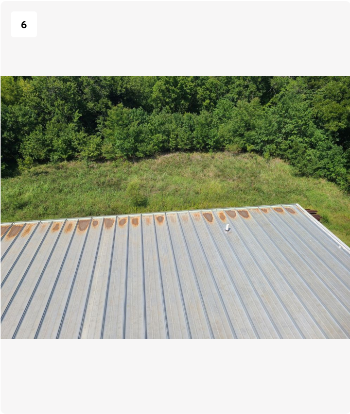
YELLOW Rust at building edge
